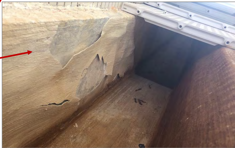
Competition Pool Gutter – walls are bulging and deteriorating
